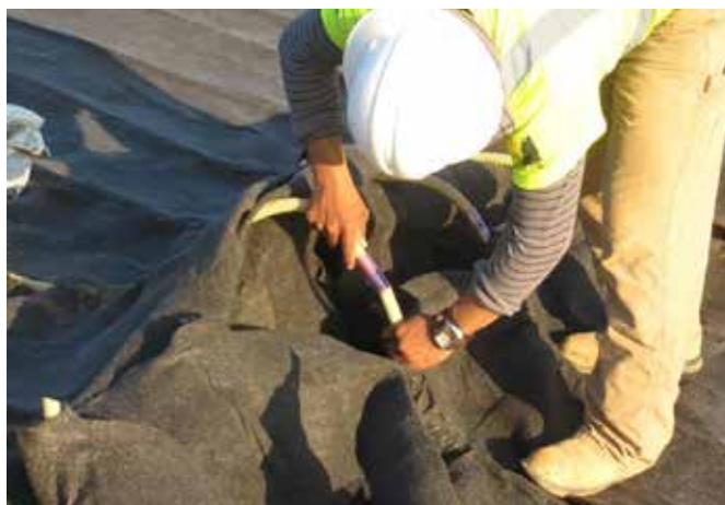
Figure 7: Mini-pipe junction with couplers
